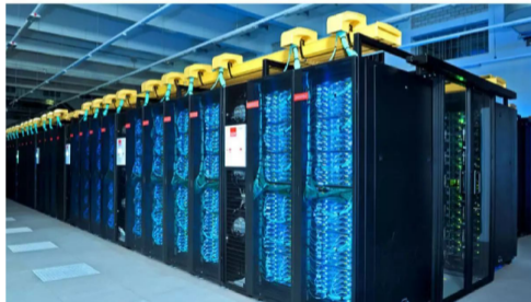
Leibniz Supercomputing Centre, Germany
